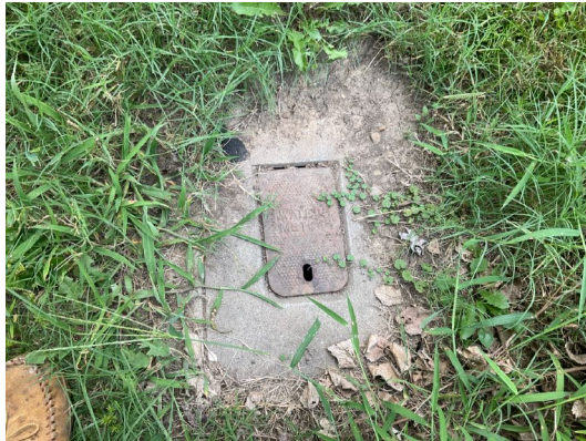
Water Meter/Water Shutoff
