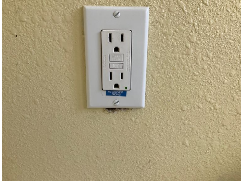
Bathrooms GFCI Protection
