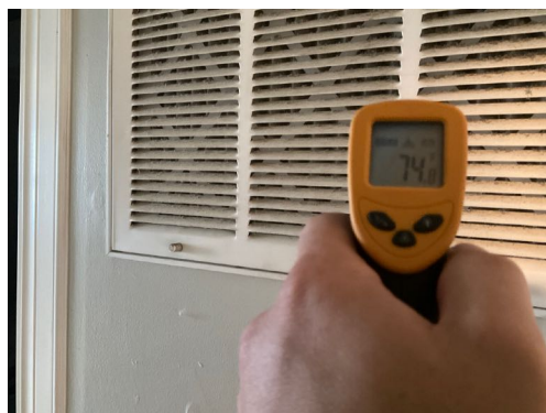
HVAC Return Temperature
