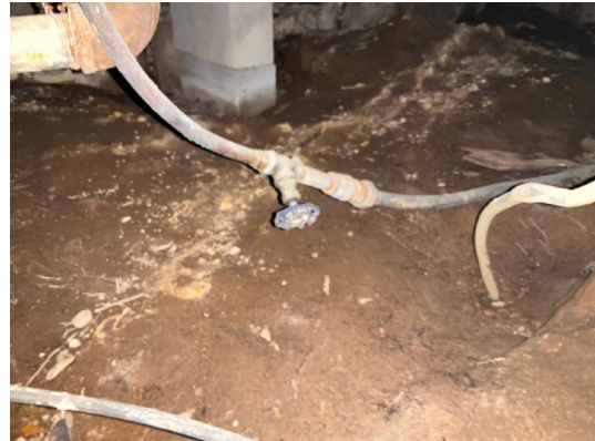
Secondary Water Shutoff
