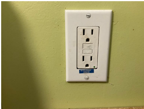
Kitchen GFCI Protection
