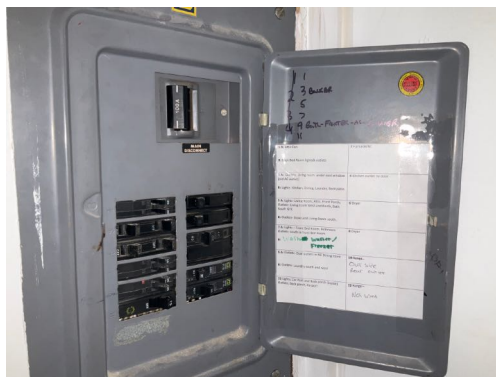
Main Panel Door Open
