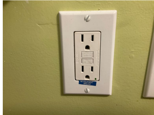
Kitchen GFCI Protection
