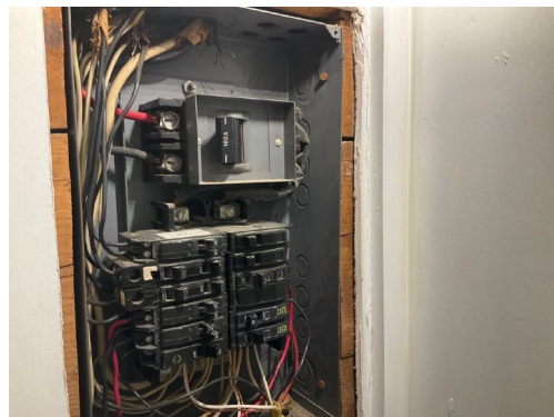
Dead Front Cover Removed
